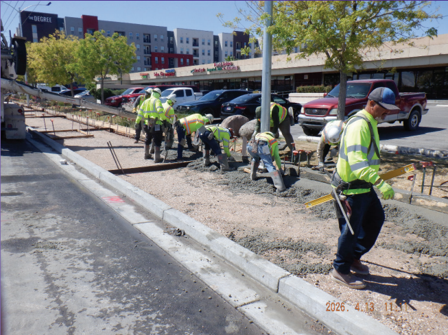
Crews pouring concrete for a new sidewalk on Maryland Pkwy, south of Flamingo Rd.
